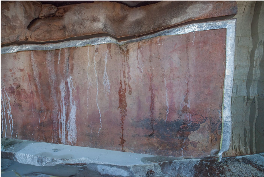
Figure 16. Breaching of waterproofing caused by a defective silicone seal and the accidental breaching of the plastic. The slurry was immediately removed and there is no permanent damage to the rock art.
